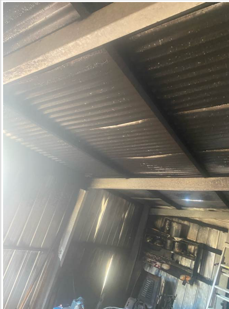
Smoke / soot damages to internal shed
