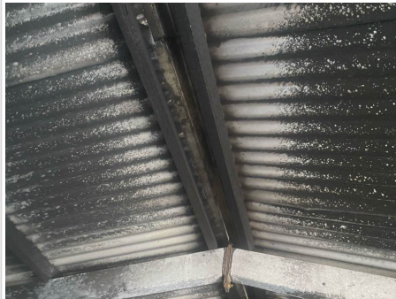
Fire damaged roofing sheets and battens
