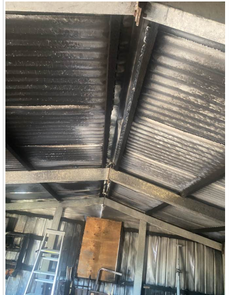
Internal fire damages
