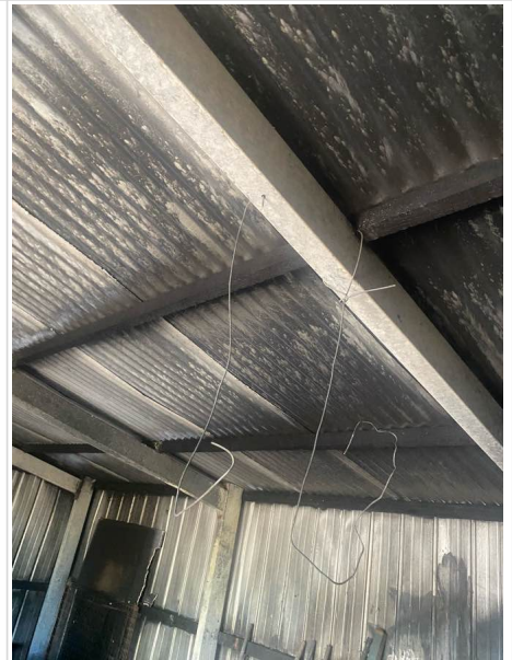
Damaged roof battens and roof sheets
