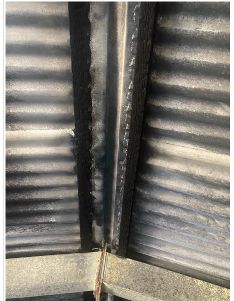
Burnt timber roof battens
