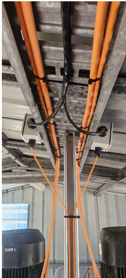
Figure 3: Existing Cabling and Tray to be Reinstated in New Shed
