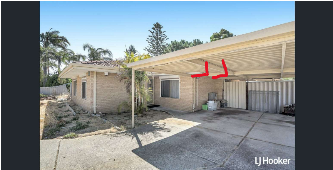
Figure 6 My suggestion would be to bolt some kind of L shaped metal flush against the external wall and bend it around the gutter and up wards to support the highest side of the skillion slop.
